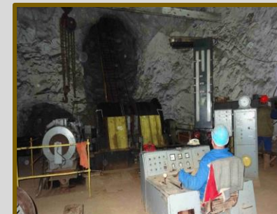
Underground hoist chamber
