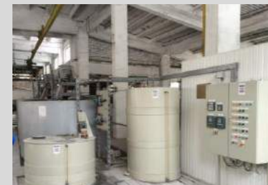
Processing plant comprising crushing, milling and flotation circuits
